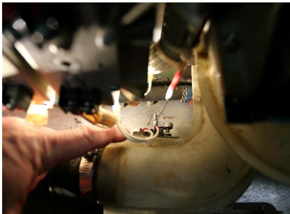
FIGURE 8-10: HEATER DUCT SWITCH
